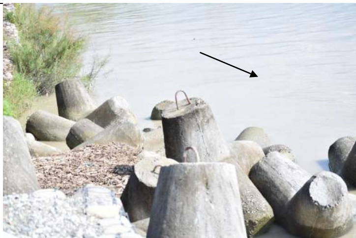
Figure 10.5 Vortex breakers provided on the right bank of the Sharda river upstream of Tanakpur Barrage
