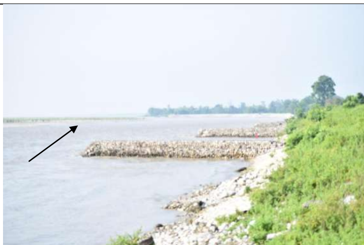
Figure 10.1 Series of spurs provided on right banks of Sharda river downstream of the Banbasa barrage
